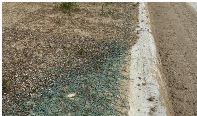
6. A competitor's inferior excelsior blanket failed to contain sediment, allowing runoff into the street and creating cleanup costs and potential fines. The fibers in this blanket do not expand or perform like Curlex fibers.
