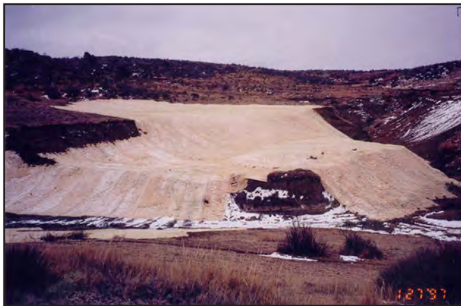
Excelsior ECBs on Utility Slope Surface Stabilization Project in 1997. Photo courtesy of American Excelsior Company.
