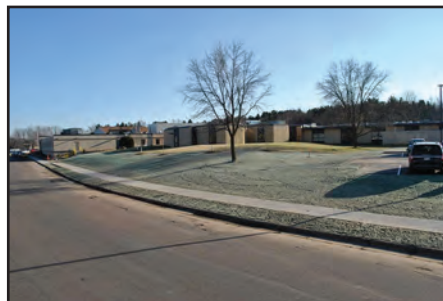
Hydraulically Applied Erosion Control Product (HECP) Application. Photo courtesy of American Excelsior Company.
