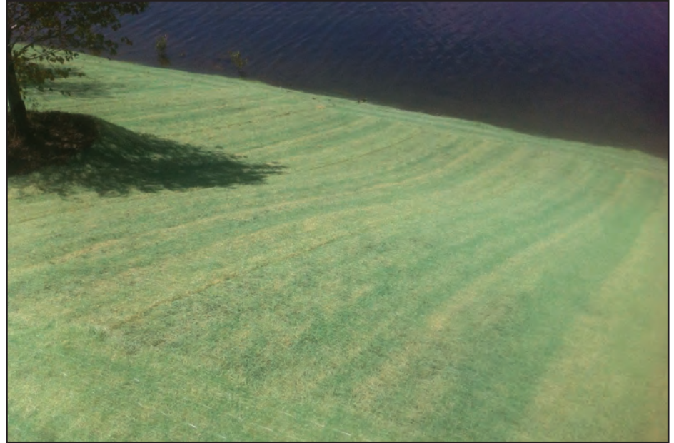
Dyed Green Excelsior ECBs offer a “finished look” to slope surface stabilization ECB applications. Photo courtesy of American Excelsior Company.
