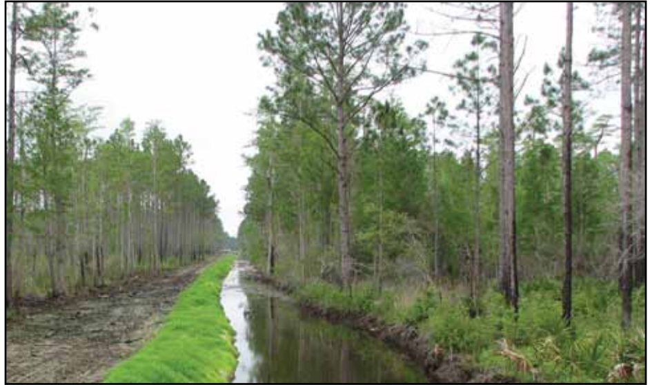
Vegetated erosion control blankets protecting bank a few weeks after installation (left side of photo).
