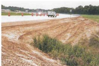
Prior to installing CurlexGRASS, the shoulder subgrade is properly prepared and seeded.
