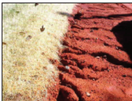
Rills formed in the soil where surface covers were not installed.
