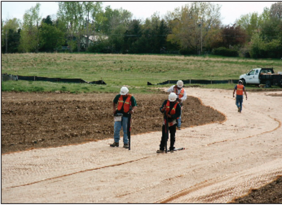
Staples were installed by the crew using a manual gun round-top pin system.
