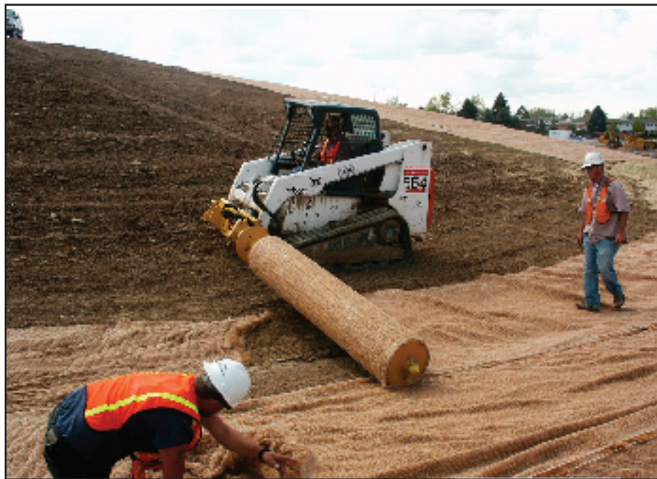
Slopes up to 2H:1V and the channel bottom were protected with a coconut fiber erosion control blanket.
