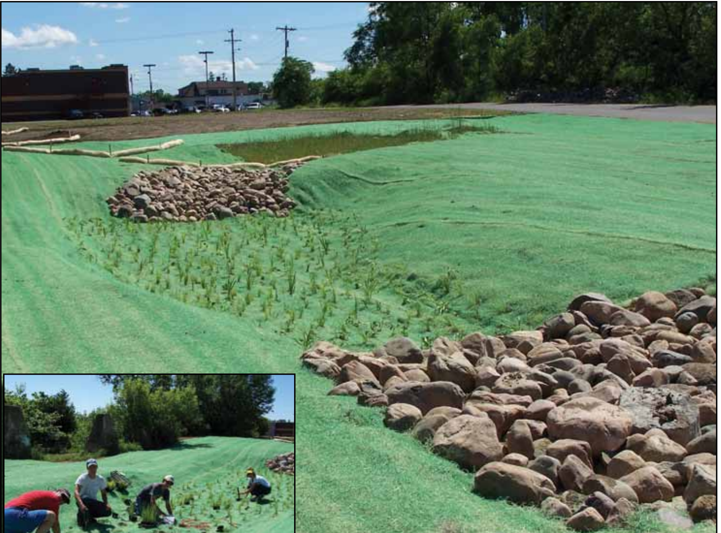
Completed raingarden system with porous excelsior fiber logs up gradient for filtering of runoff. Inset: Volunteers plugging natives through erosion control blanket (dyed green) in raingarden system. (Photos by Cooper Engineering)
