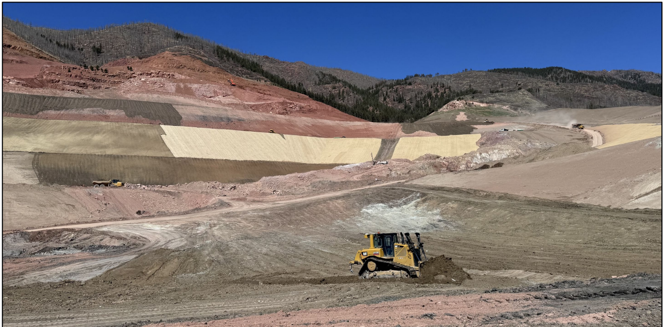
Figure 6: Landscape view of a section of the project with active grading occurring in the foreground and Curlex II FibreNet ECB installation in the background.
