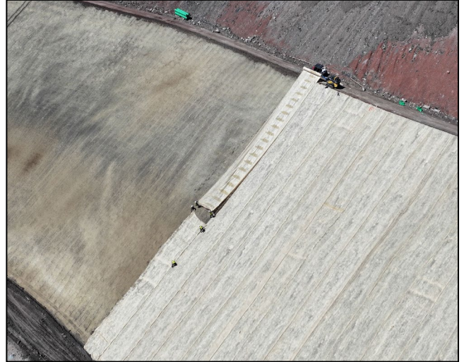
Figure 5: Aerial view of Curlex II FibreNet installation on one of the mountain slopes.
