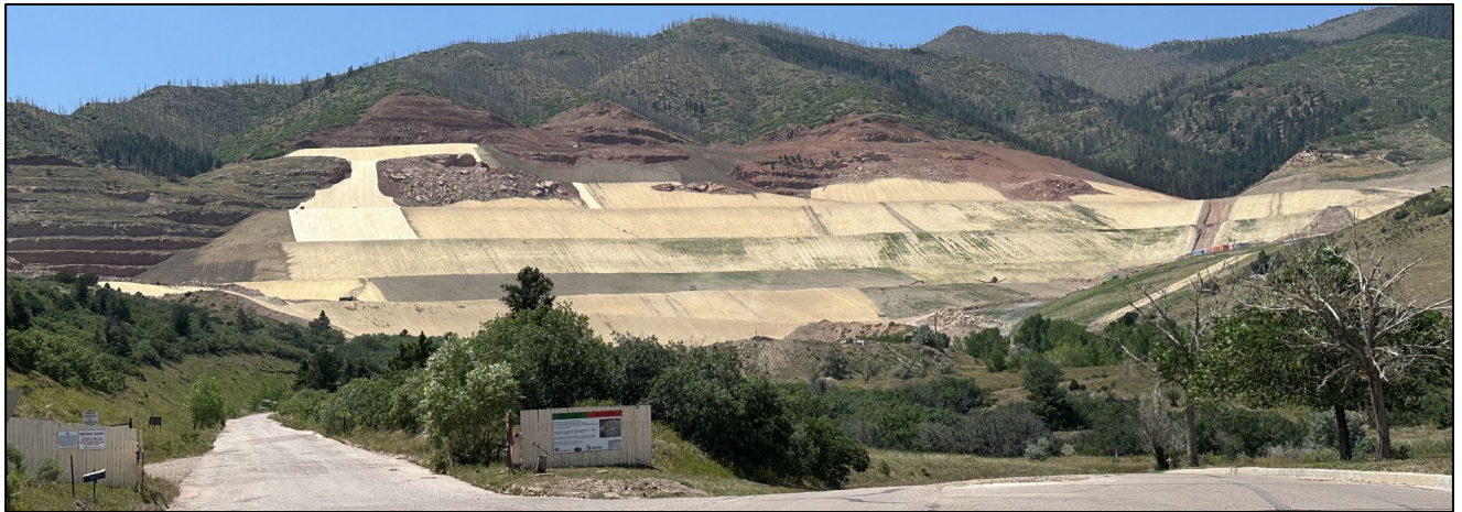
Figure 7: Landscape view of the Quarry site once all ECB installation had been completed.
