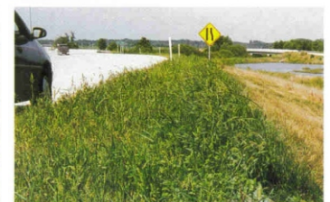
After Curlex I QuickGRASS installation, vegetation is established and the shoulder is protected.
