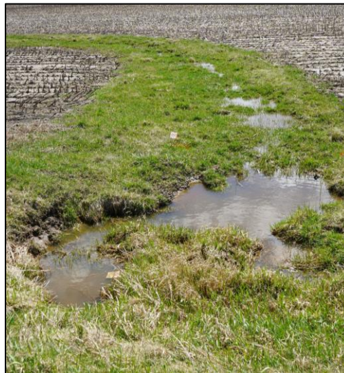
Figure 2: Surface view of one of the swales before excavation. The standing water from a prior precipitation event illuminates voids in the subgrade that resulted from years of erosion.
