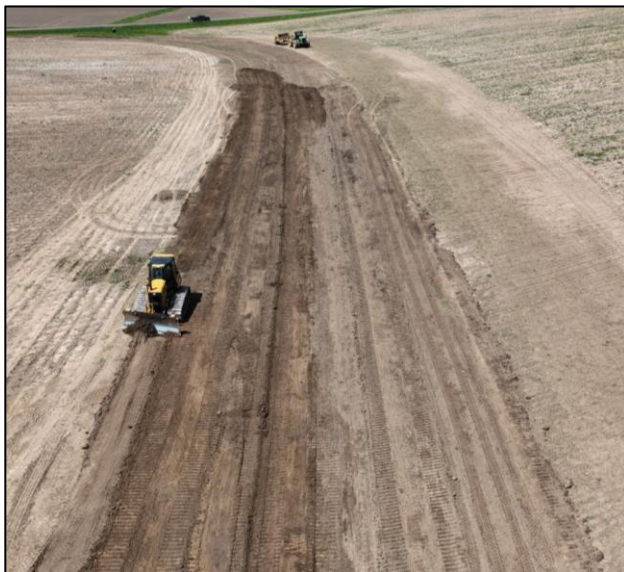
Figure 4: Heavy equipment performing grading work to widen one of the swales after its vegetation was cleared.
