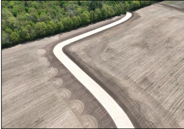
Figure 8: Aerial view of one of the swales shortly after Curlex II ECB installation (photo taken in late spring).
