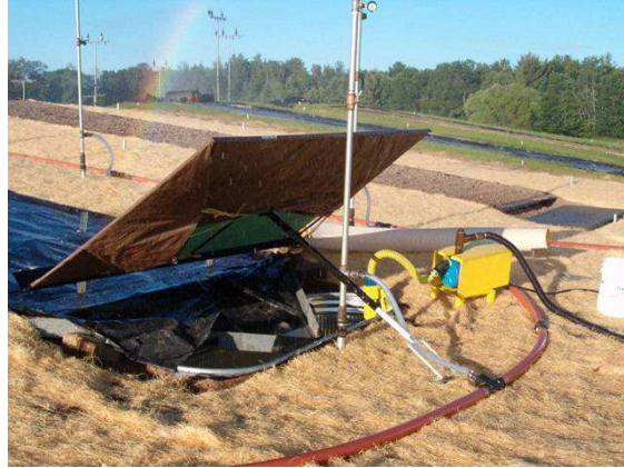
Figure 9. Collection device at toe of slope. Notice buried collection tank and evacuation pump. The collection device will ensure capture of all soil and water that will exit the plots during product testing.
